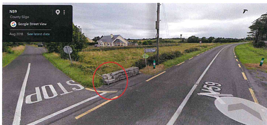
Photograph F3: The bridge wall beside the N59 at Joyce's Cross, with damage again in 2018 circled. Source: Google Street View, August 2018.
