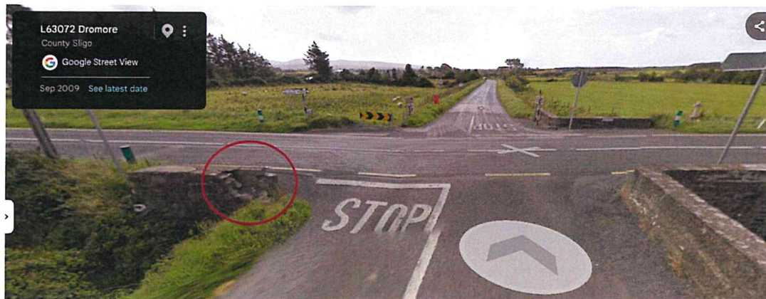
Photograph F1: Joyce's Cross viewed from the L63072, looking across the N59 towards the L2702, with damage to the bridge wall circled. Source: Google Street View, September 2009.
